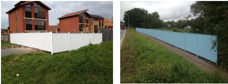
Above Left: SPS In ground Job in Nottingham, right: Weighted system at Cambridge University.
